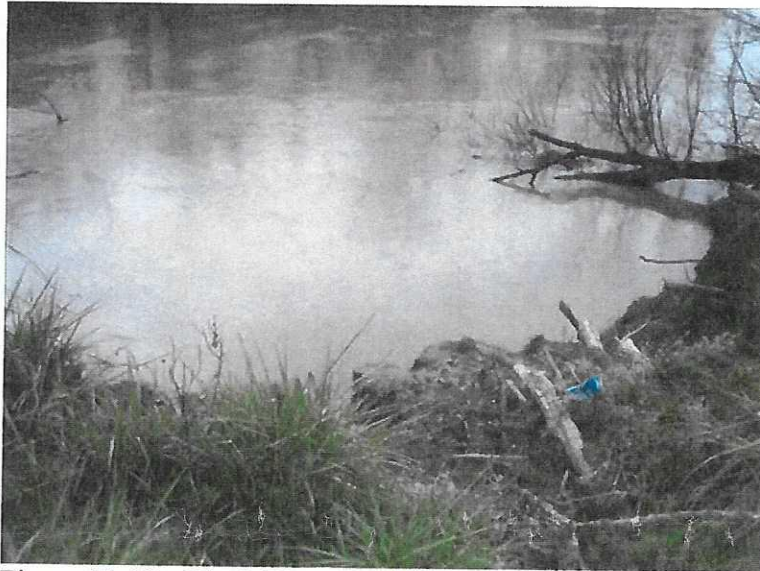
Figure 11: Big Black River Bank Erosion at the Facility
