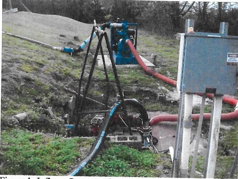
Figure 1: Influent Pumps and Permanent Influent Bypass
