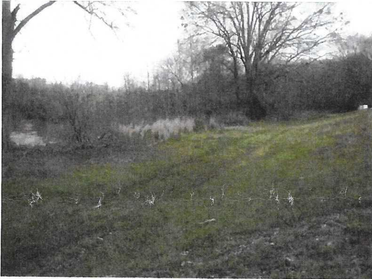
Figure 10: Distance of the Bank Erosion from the Facility's Levee.
