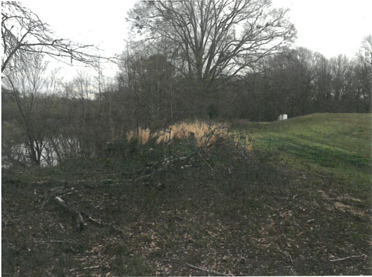
Photo taken in March 2017 shows how close the river bank soughing is to the toe of the lagoon levee.
