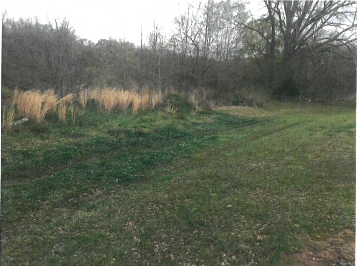
Photo taken in March 2017 shows how close the river bank soughing is to the toe of the lagoon levee.
