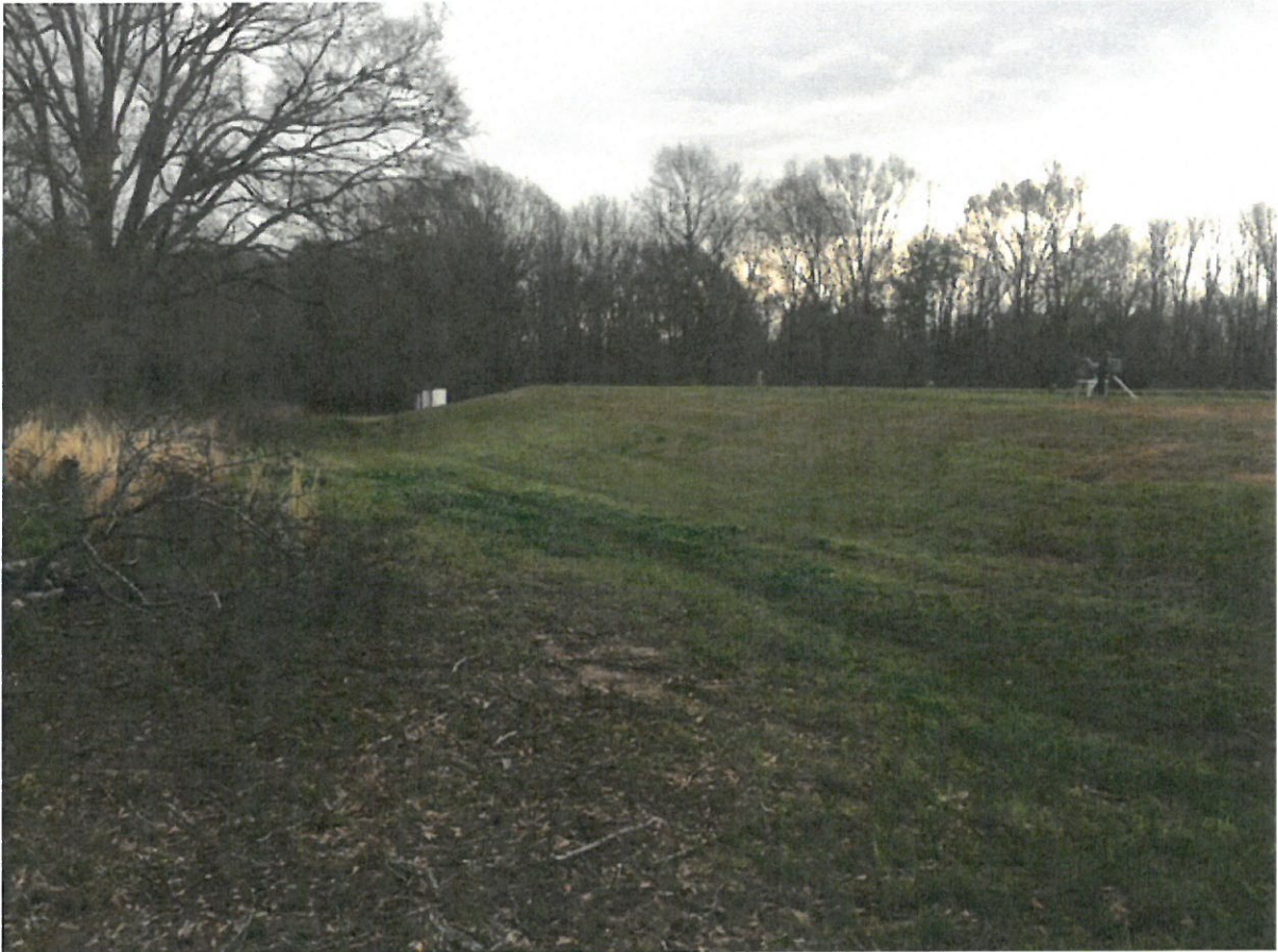
Photo taken in March 2017 shows how close the river bank soughing is to the toe of the lagoon levee.
